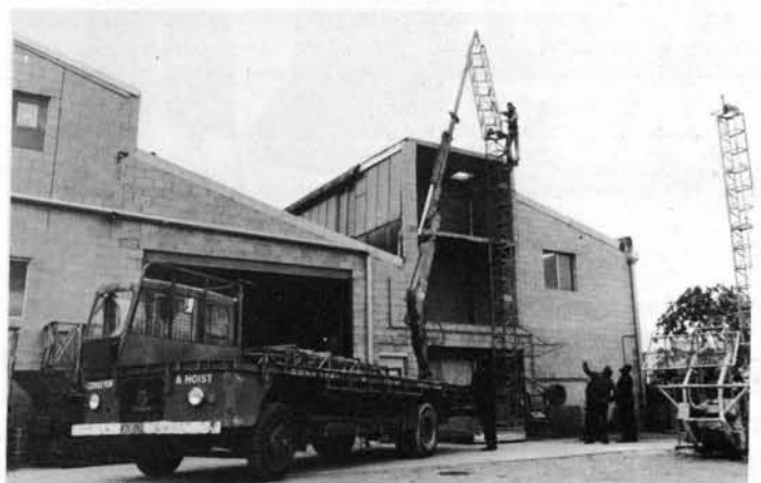
Truck mounted cranes enable drivers to erect, rig and service hoise towers.
