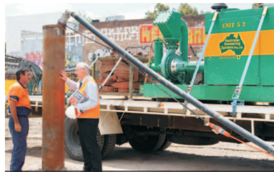
Aussie Pumps Neil Bennett with Steve Newland check out the installation of Tsurumi KTZ submersibles
